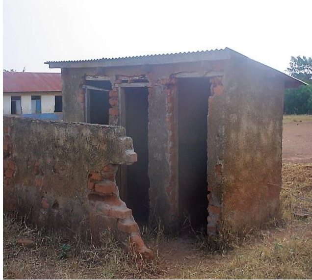
Photo 3: Latrine in poor structural condition with missing components (Source: Field Survey, 2025)
