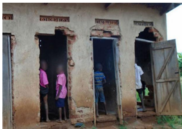
Photo 1: Latrine block with broken door and deteriorating walls (Source: Field Survey, 2025)
