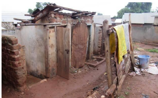
Photo 2: Non-segregated latrine cubicles lacking privacy infrastructure (Source: Field Survey, 2025)
