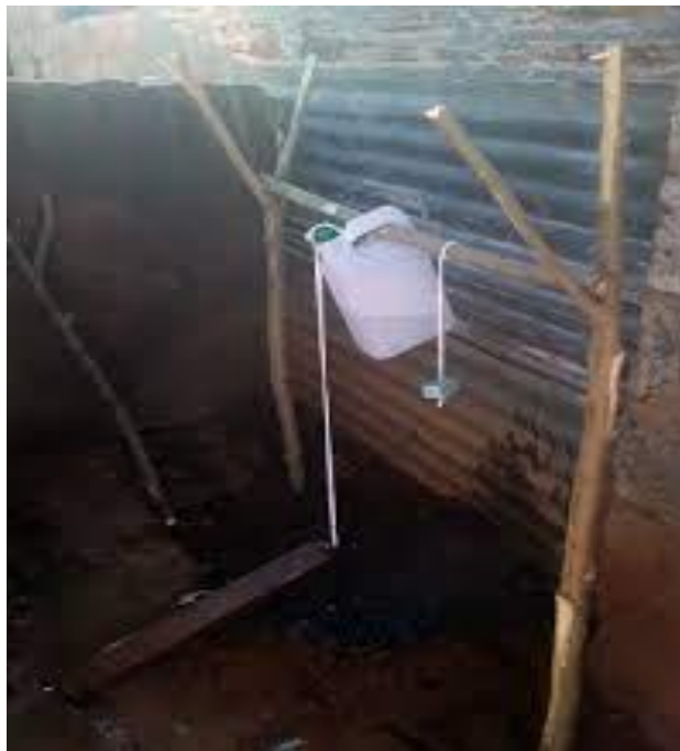
Photo 4: Deteriorated handwashing station without soap or clean water (Source: Field Survey, 2025)
